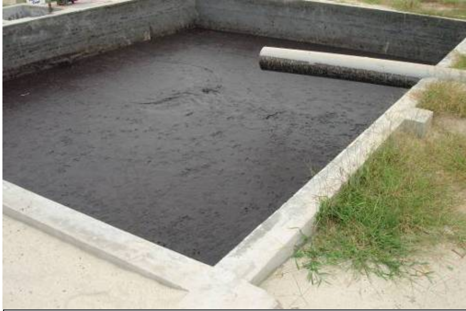
Sludge Drying Bed
